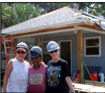
Volunteers and a future homeowner working on our newest rehab project in Jax Beach.
